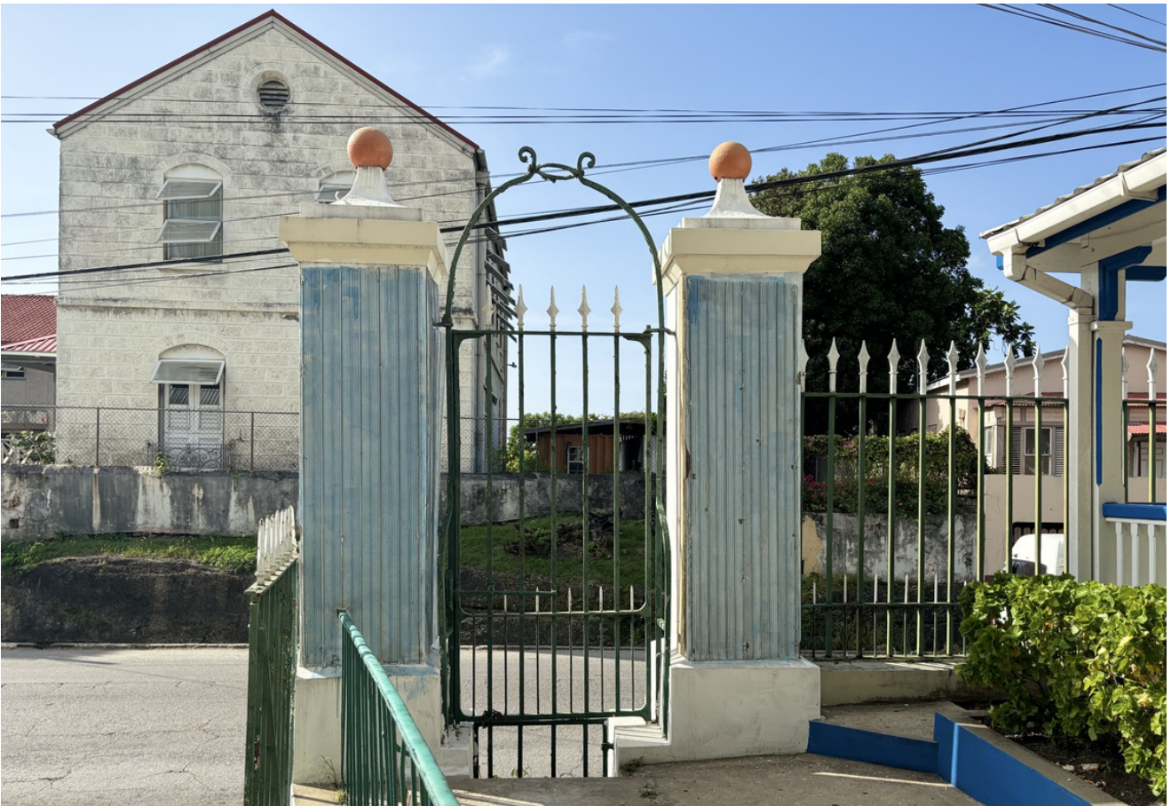
A closer view of the preparatory work on the Queen's gate columns.
