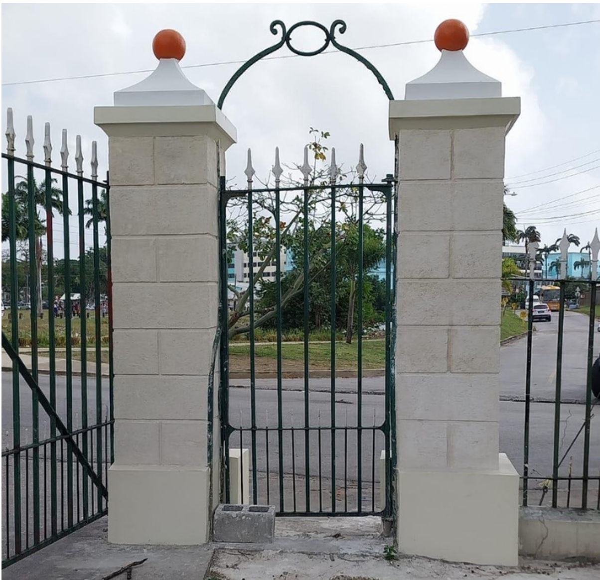
A closer view of the coral rendered columns at the President's gate.
