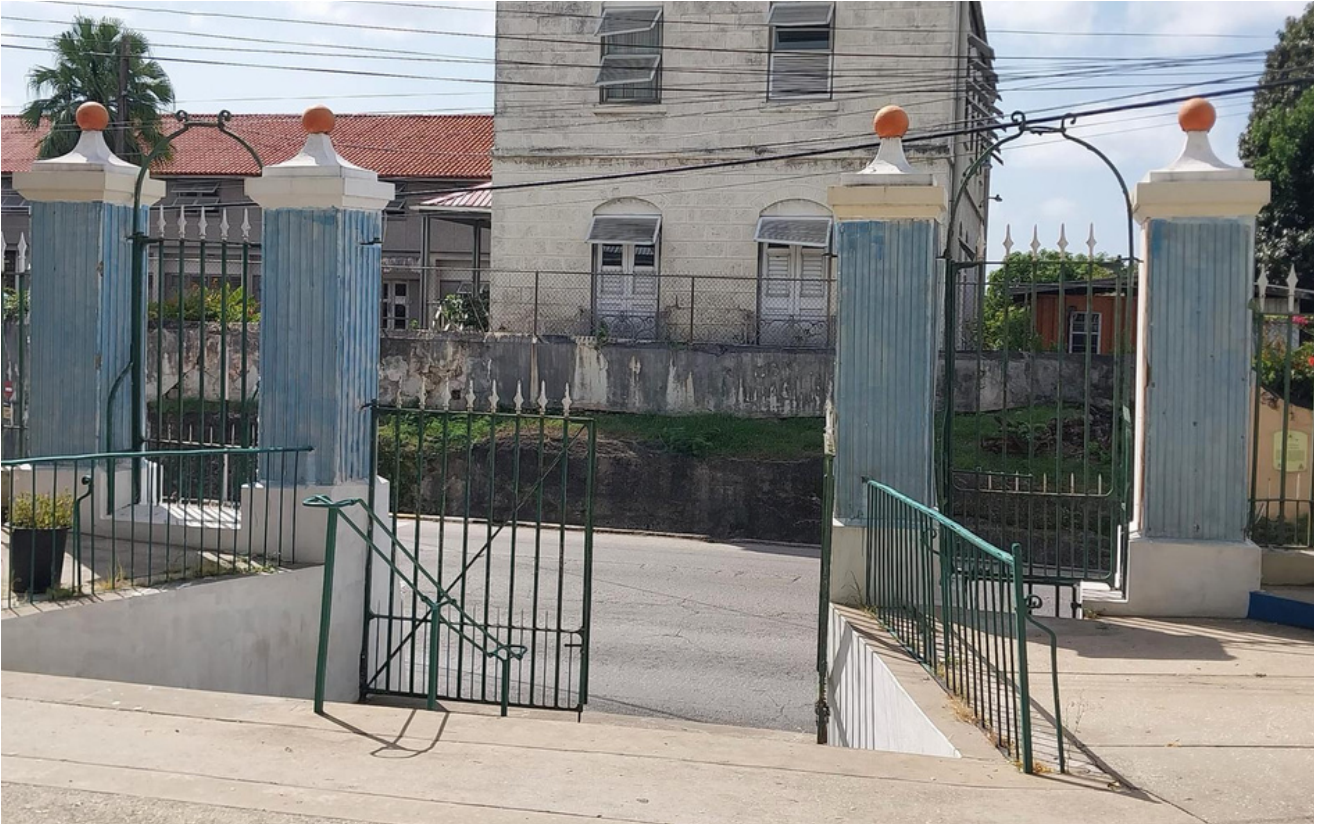
Full view of the preparatory work on the Queen's gate columns in Queen's Park.
